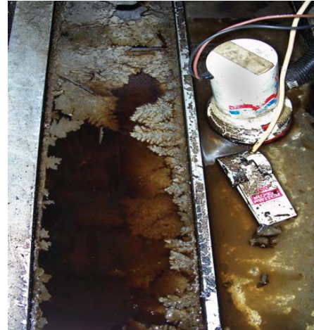
The use of a bilge sock would help prevent oil collected in the bottom of this bilge from being discharged to the marine environment
